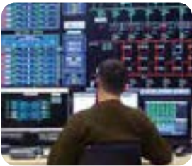
Command and Control Rooms
